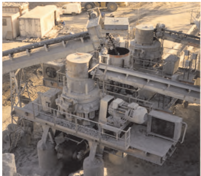
Plant with DUSTEX® in operation
